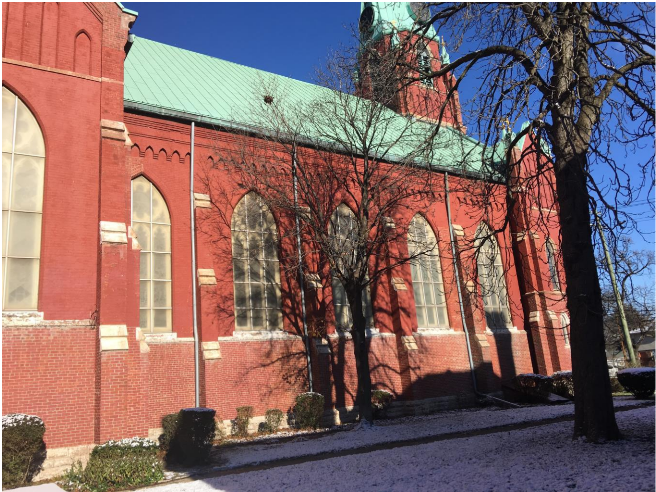
Image 5: The southeast side of the church has several downspouts; some are disconnected and some may be connected. These would be directed to proposed Practice 4.
