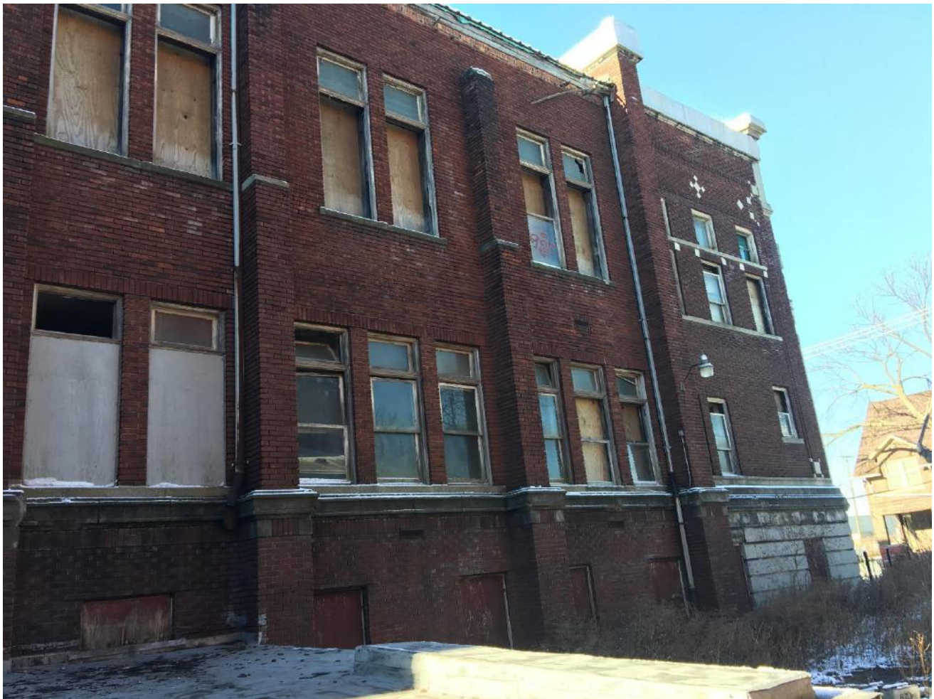
Image 2: The west side of the abandoned school building. Some downspouts appear to be missing (such as the one in the foreground) and some still look connected (background). The runoff from this portion of the building would be directed to proposed Practice 2.
