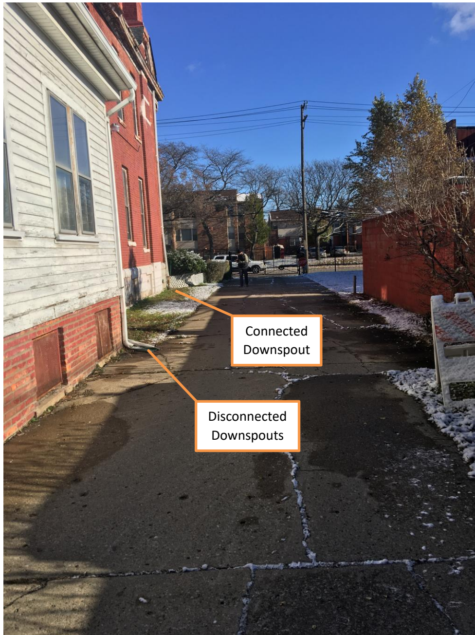
Image 7: Disconnected downspouts and connected downspouts are both found on the property, as shown here on the rectory. If a shared practice was implemented with Joseph Frontera & Son, it could be located to the right of the pictured driveway.
